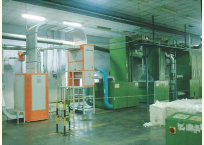
THE VISION SHIELD-FROM JOSSI-SWITZERLAND, Installed in blow room.
